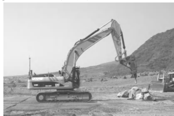
Fig7 Operational limits in remote operation (breaker)
